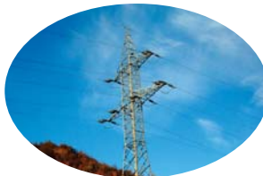
Daily, RAIGI connects you to the electricity network
